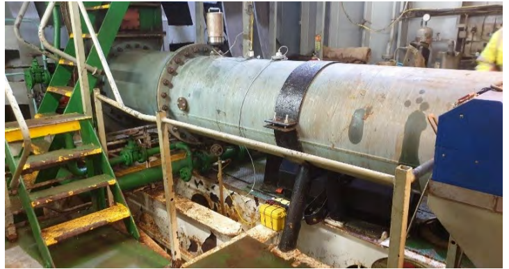
Sensor on pipe
